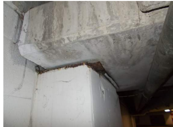
Photo 5.02 Surface corrosion on steel bearing plate
