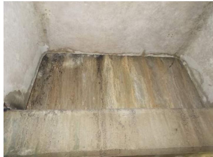
Photo 9.01 Efflorescence and staining on side of inverted tee
