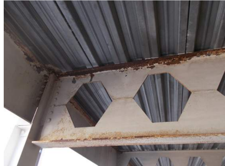
Photo 10.02 Corrosion on steel framing
