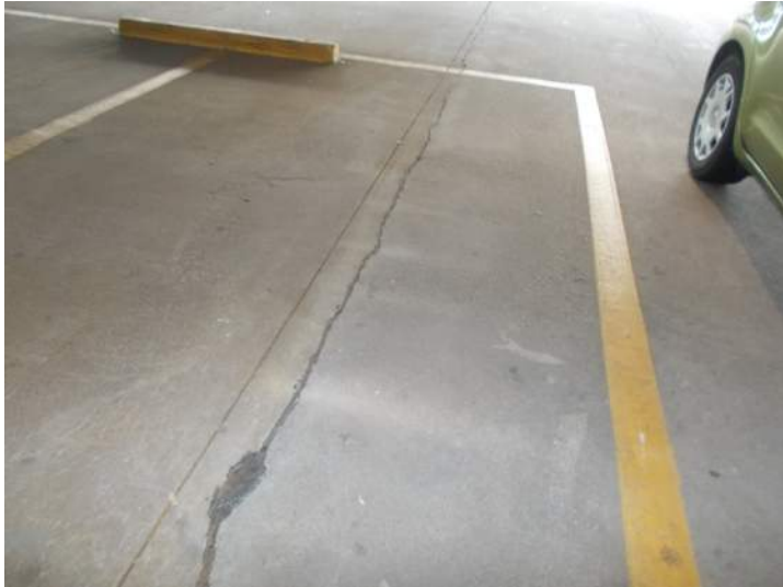
Photo 7.01 Wide joint in garage slab
