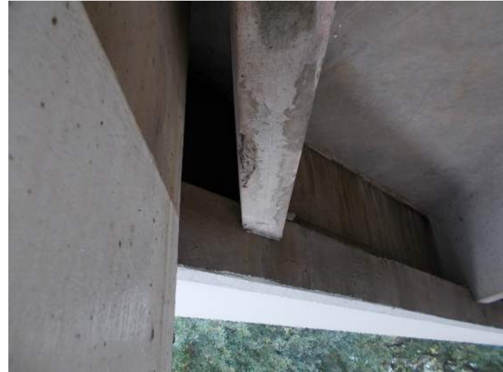
Photo 11.02 Spall in double tee stem
