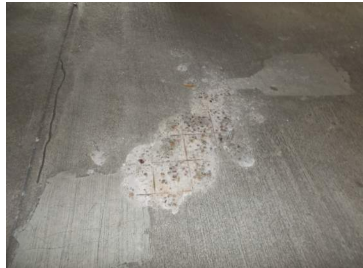
Photo 12.01 Exposed welded wire fabric at top of slab
