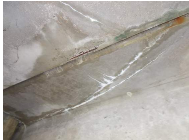
Photo 6.04 Crack with efflorescence in flange
