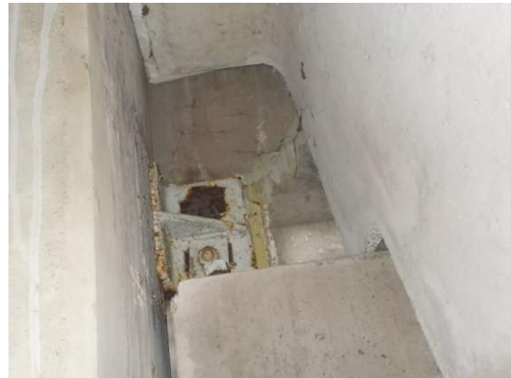
Photo 1.03 Damaged spandrel to column connection
