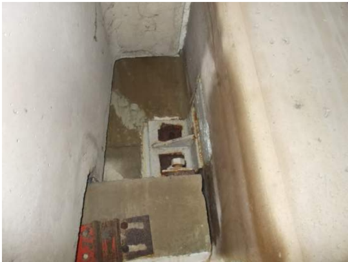
Photo 1.01 Broken spandrel to column connection
