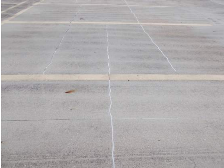
Photo 17.01 Long cracks in upper deck
