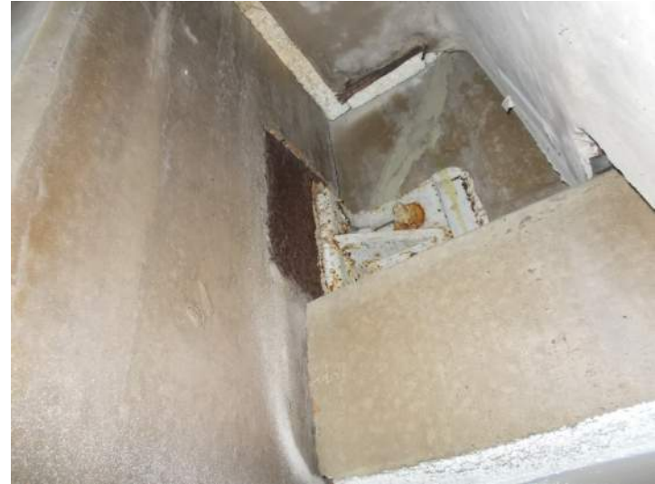
Photo 3.01 Corrosion at spandrel connection
