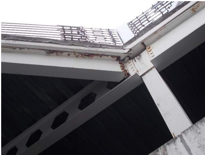
Photo 10.01 Corrosion on steel framing
