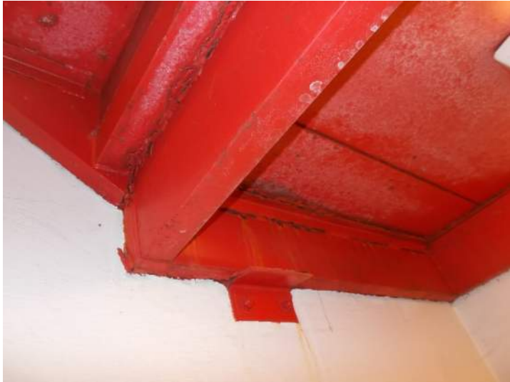
Photo 19.02 Corroded stair framing
