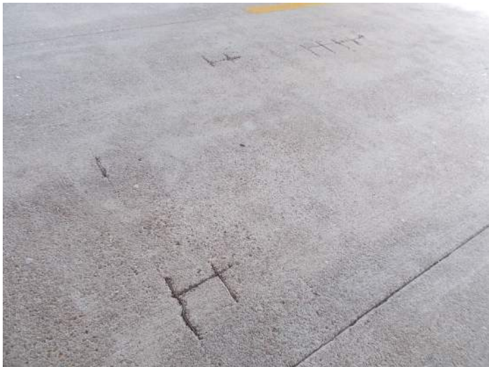
Photo 12.03 Exposed welded wire fabric at top of slab
