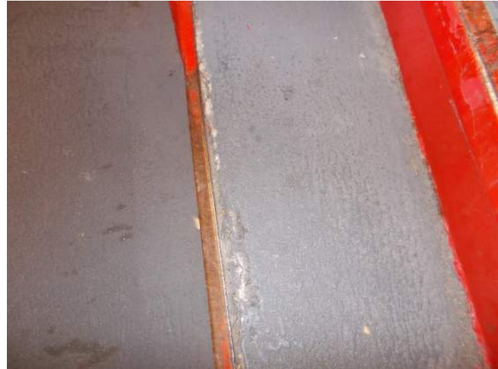
Photo 18.02 Detached nosing on stair
