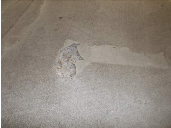
Photo 12.02 Exposed welded wire fabric at top of slab
