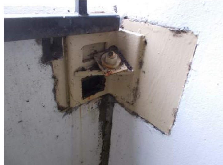
Photo 1.02 Broken spandrel to column connection
