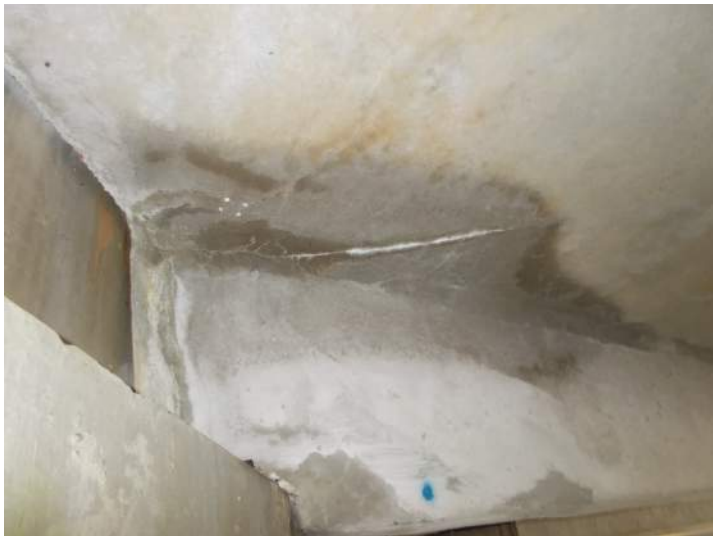
Photo 6.02 Crack with efflorescence at stem to flange interface
