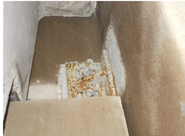
Photo 3.02 Corrosion beginning at spandrel connection
