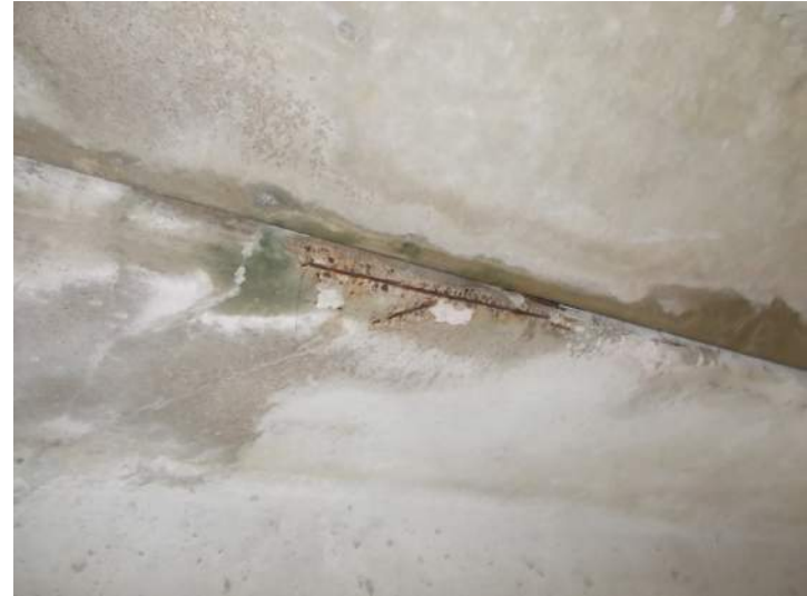
Photo 8.01 Minor spalling/low cover for reinforcement
