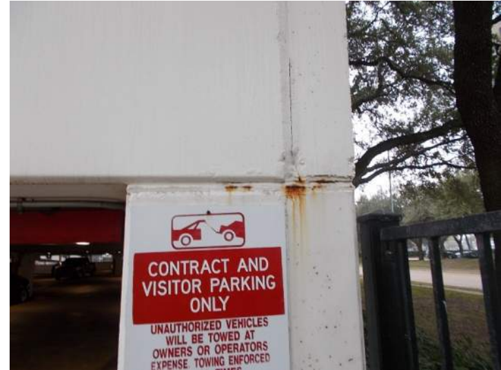
Photo 5.01 Rust staining at steel bearing plate
