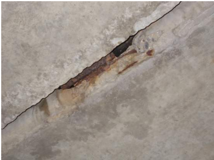
Photo 4.02 Corrosion and spalling at flange tip connection
