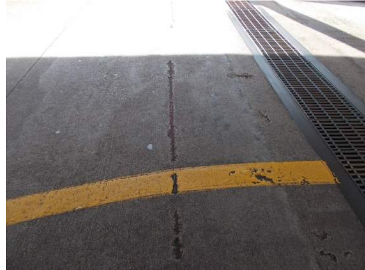
Photo 12.04 Exposed rebar at top of slab
