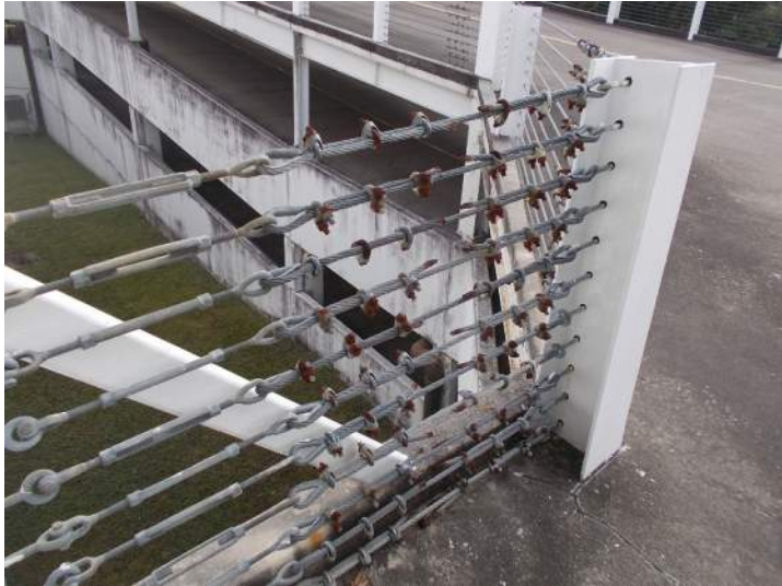
Photo 13.02 Surface corrosion on cable barrier connectors
