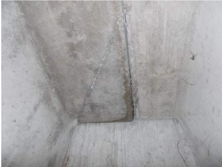
Photo 6.01 Crack with efflorescence in flange
