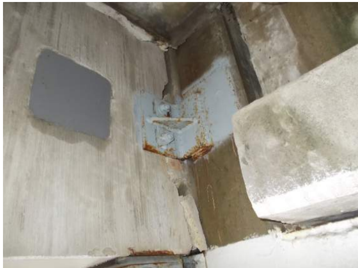
Photo 2.01 Broken panel at spandrel connection
