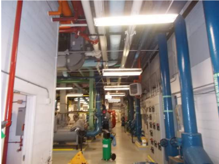
Photo 0.09 General view inside central utility plant
