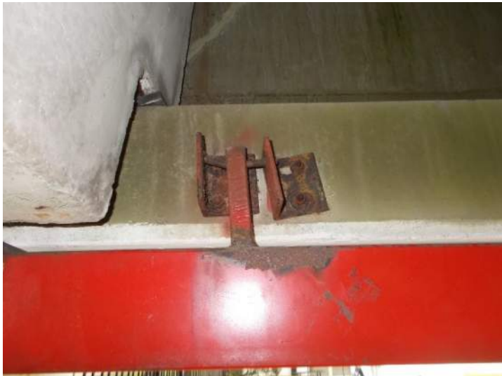
Photo 14.01 Damaged bracket supporting clearance bar
