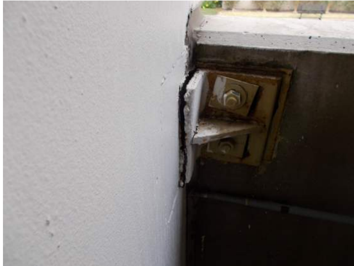
Photo 1.04 Broken weld spandrel to column connection
