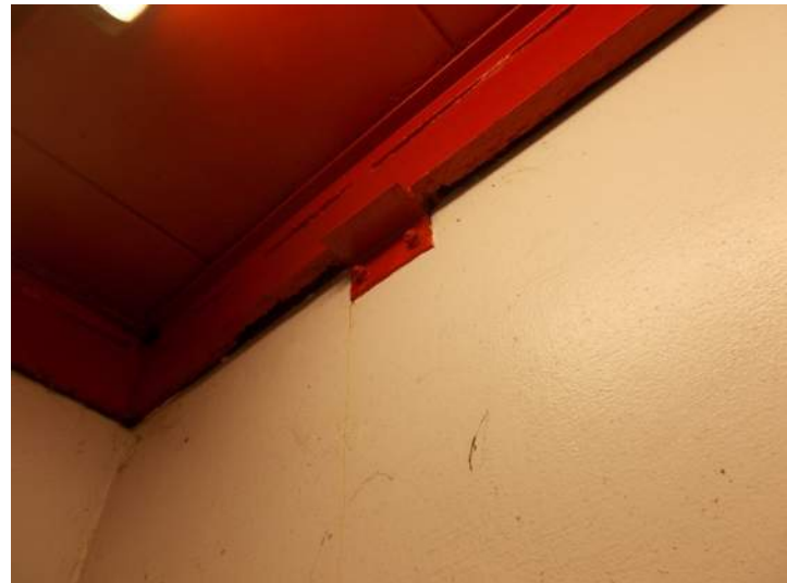
Photo 19.01 Corroded stair framing next to wall
