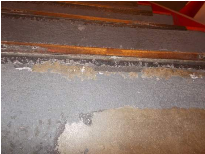
Photo 18.01 Detached nosing on stair
