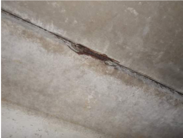
Photo 4.01 Corrosion and minor spalling at flange tip connection
