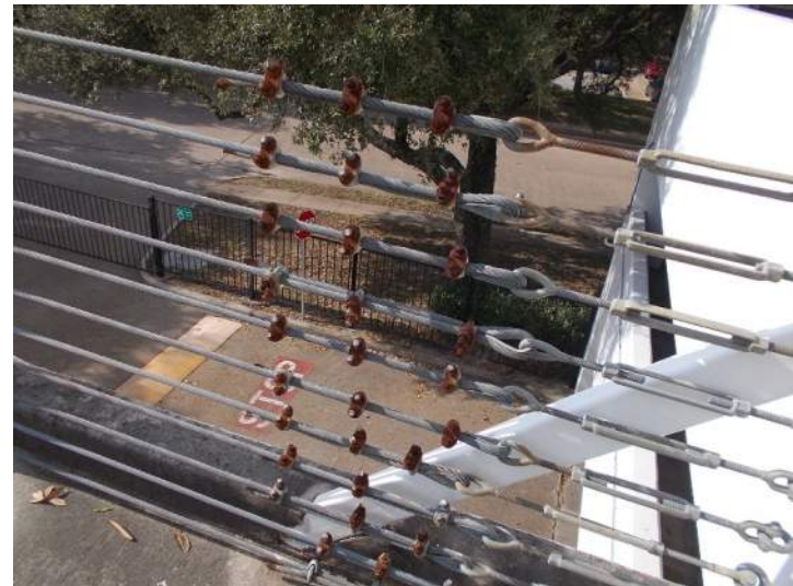
Photo 13.01 Surface corrosion on cable barrier connectors
