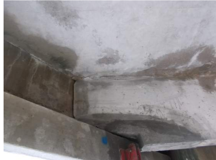
Photo 6.03 Crack at stem to flange interface
