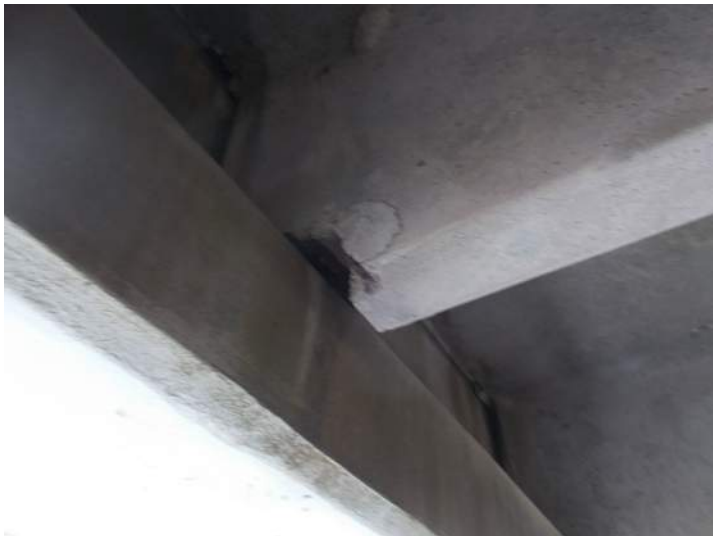
Photo 11.01 Small spall in double tee stem
