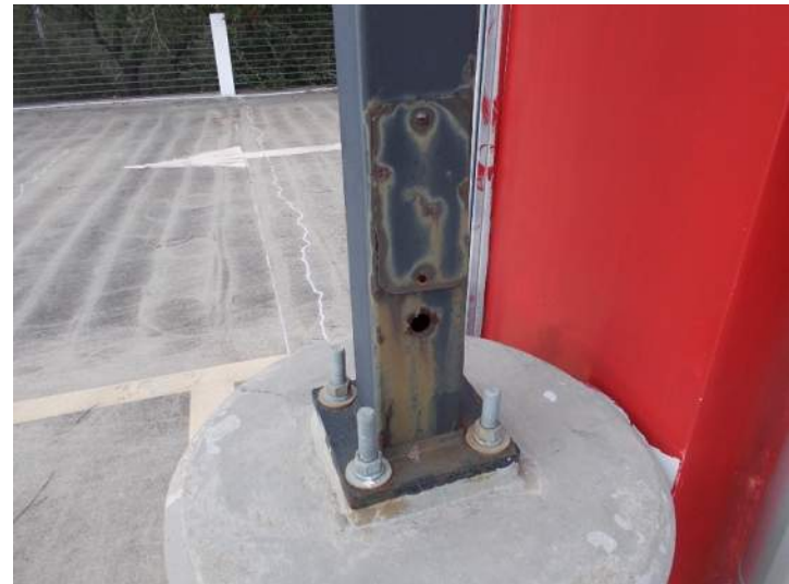
Photo 22.01 Surface corrosion on light poles
