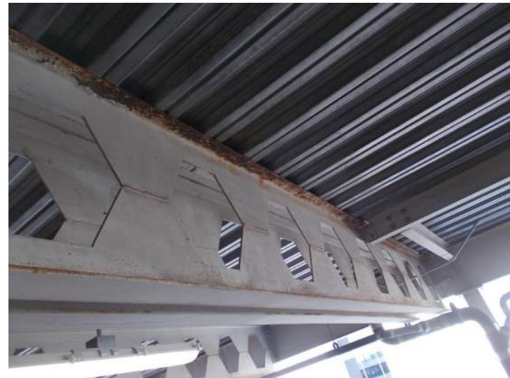
Photo 10.03 Corrosion on steel framing
