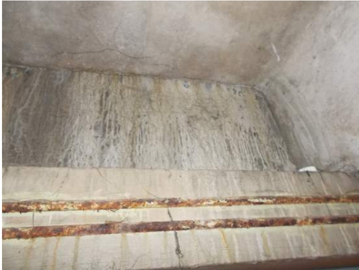
Photo 9.02 Efflorescence and staining on side of inverted tee
