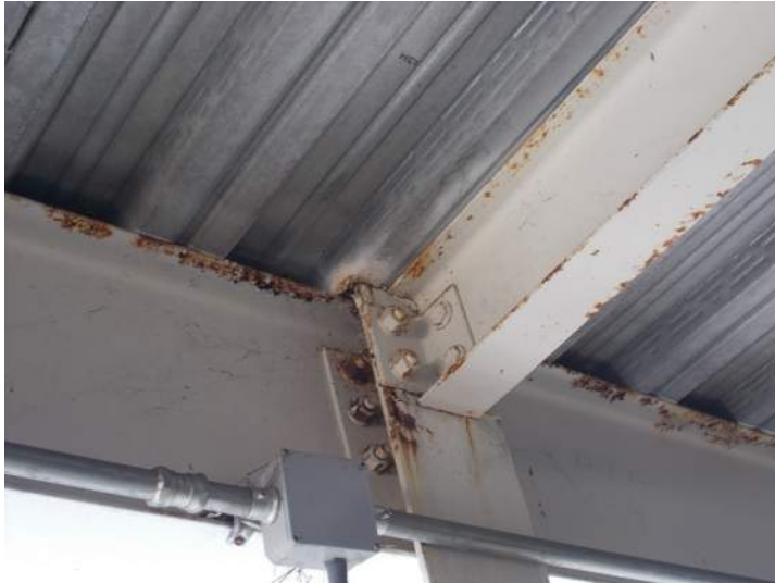
Photo 10.04 Corrosion on steel framing
