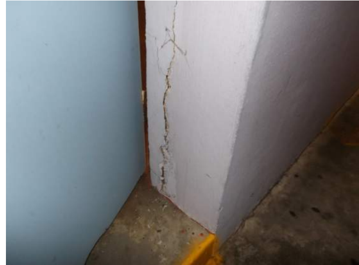
Photo 15.01 Cracked and delaminated concrete at stair
