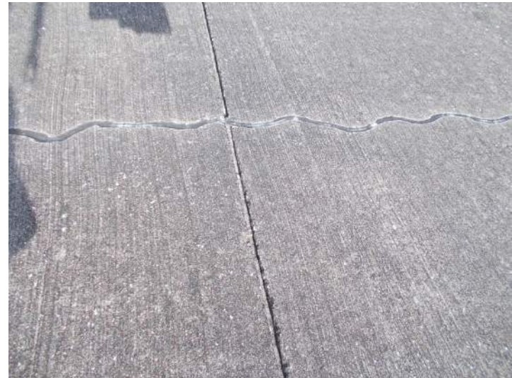
Photo 16.01 Ramp joint without sealant
